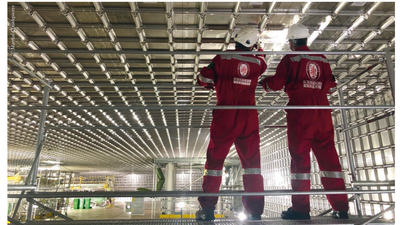
Bureau Veritas experts inspect the GTT Mark III tank during the construction of the CMA CGM JACQUES SAADE , the largest LNG-powered containership in the world.
