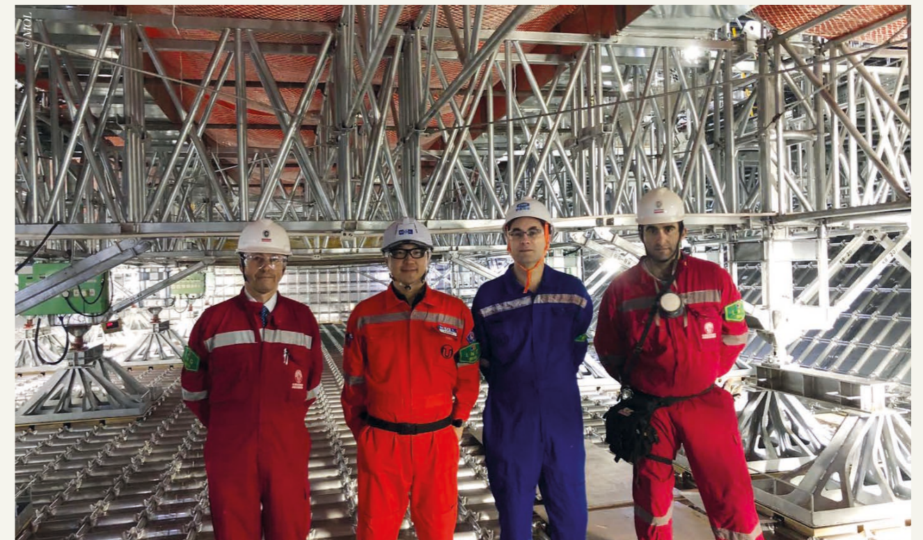
Project site team representatives inside the Gas Agility's Mark III Flex membrane tank during construction in the Hudong Zhonghua shipyard.
